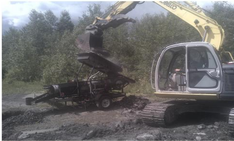
Figure 19. A view of the mobile washing plant being loaded by a small excavator.
